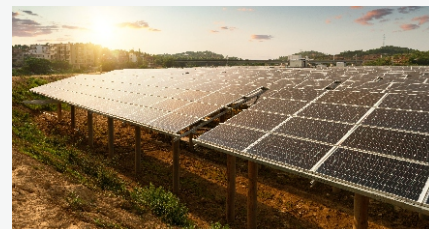
Ground-mounted photovoltaic power station
