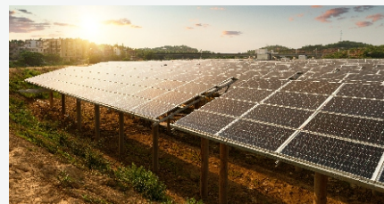
Ground-mounted photovoltaic power station
