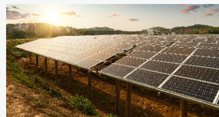
Ground-mounted photovoltaic power station
