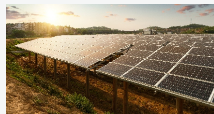
Ground-mounted photovoltaic power station
