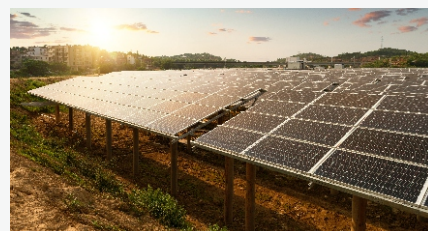
Ground-mounted photovoltaic power station
